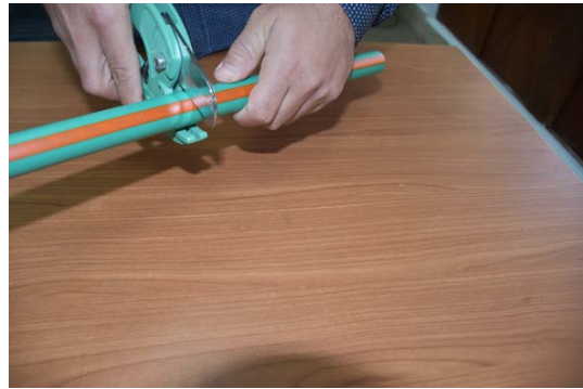
1. Pipes are measured and cut to the required length. Cutting should be rectangular to the pipe axis (90°).
